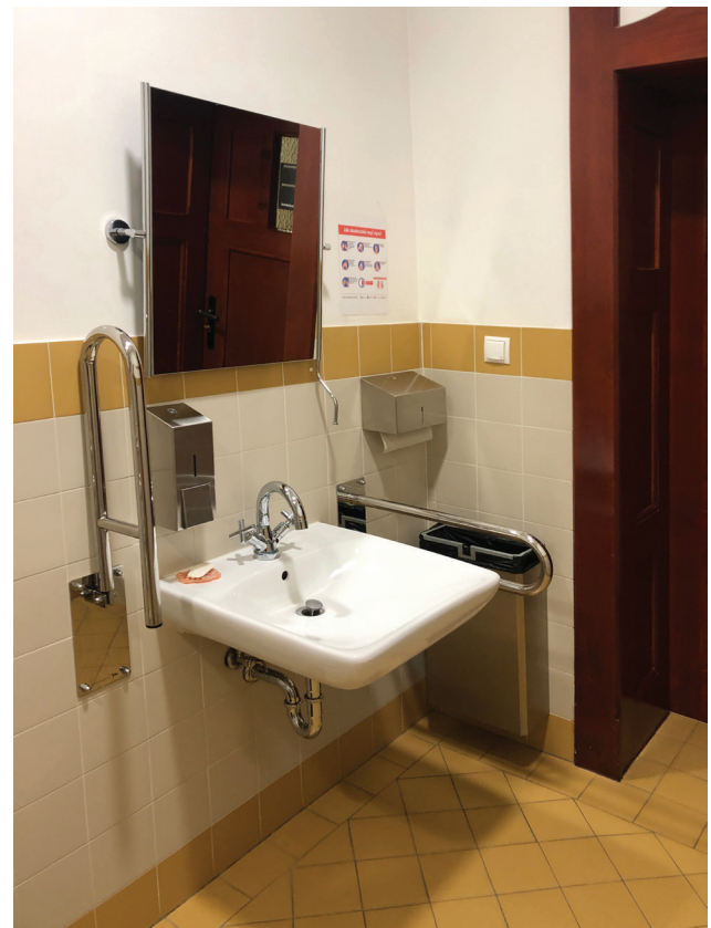
Fig. 8. Sink for disabled people in building E-5 at the Faculty of Architecture of the Wrocław University of Science and Technology
